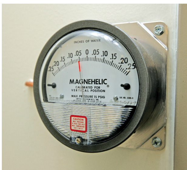
FIGURE 16. Magnehelic Gauge for Visual Confirmation of Pressurization
